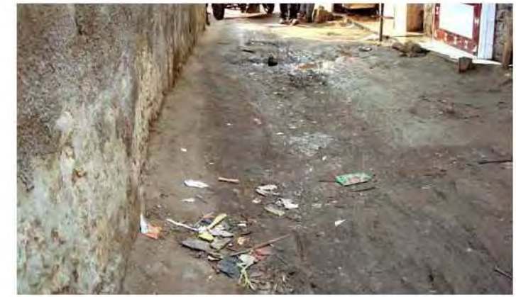
3 Asphalt in poor condition
