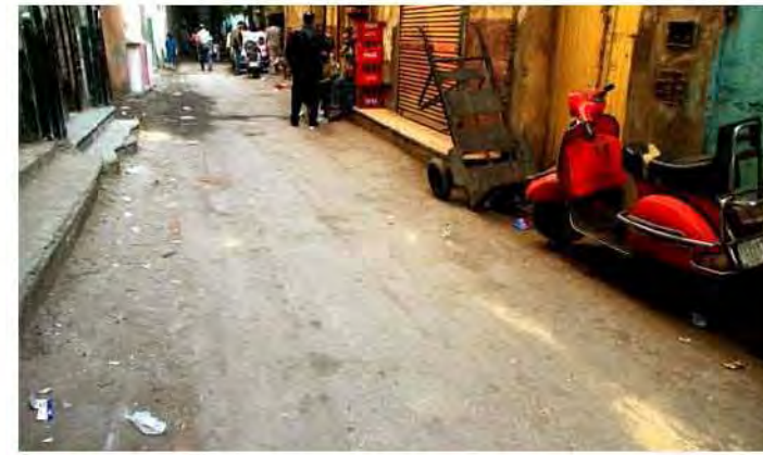
2 Asphalt in medium condition
