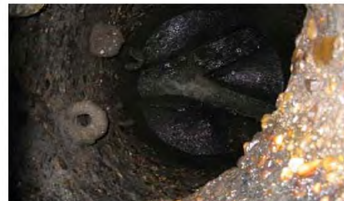
Manhole shaft in bad condition
