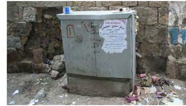
Electrical distribution box in a poor condition
