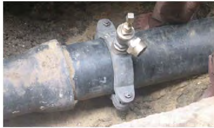
House connection fixed on a water pipe Ø160 mm
