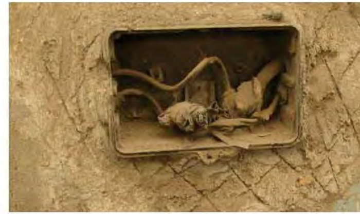
Building connection box in a dangerous condition
