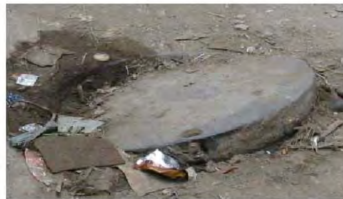
Manhole cover in bad condition
