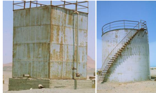
Figure 25 main steel communal water tank
