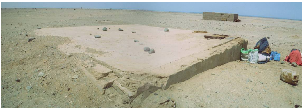
Figure 24 Communal concrete water tank
