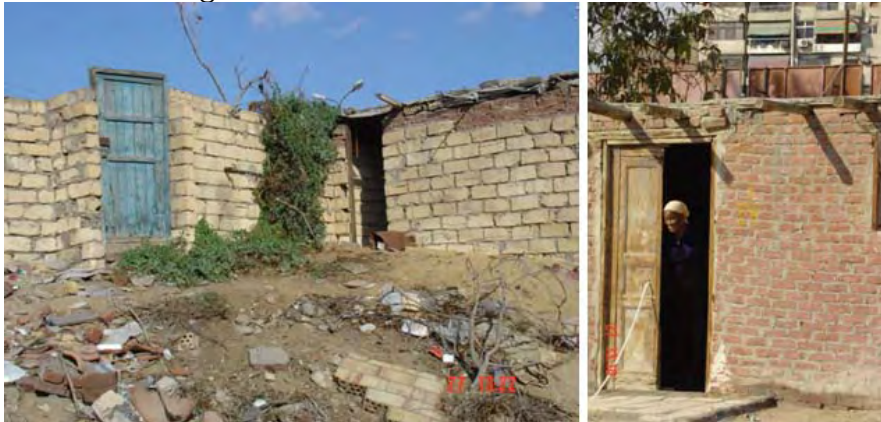
Figure 20 Buildings in bad Conditions
