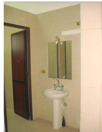
Common toilet facility
